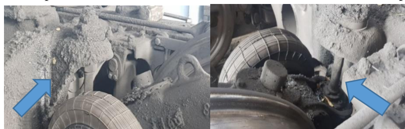
Fig. 7. Leakage of grease from the gear unit on the car ER2T 7117-08
