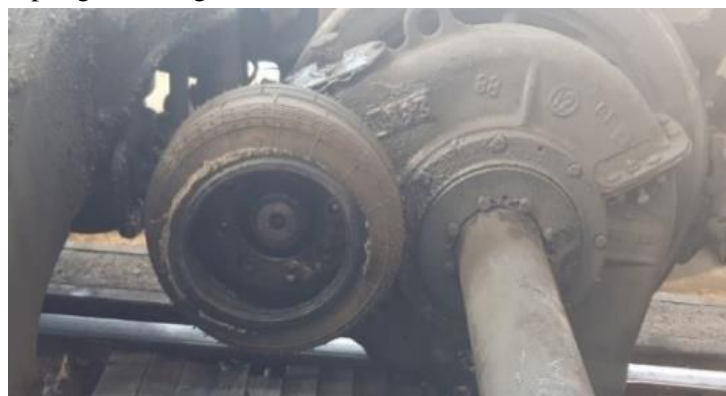
Fig. 1. ER2T car rubber-cord coupling side surface damage
